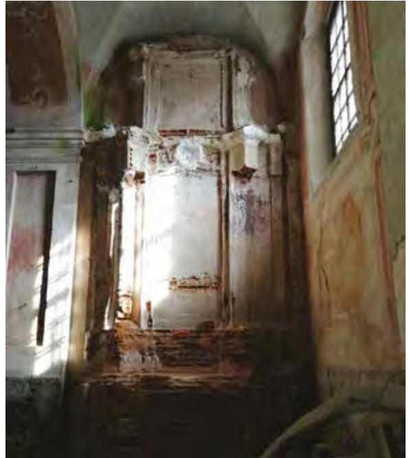
Degraded Carmelite Church in Mstislavl, Belarus, proposed for rehabilitation under COMUS program
