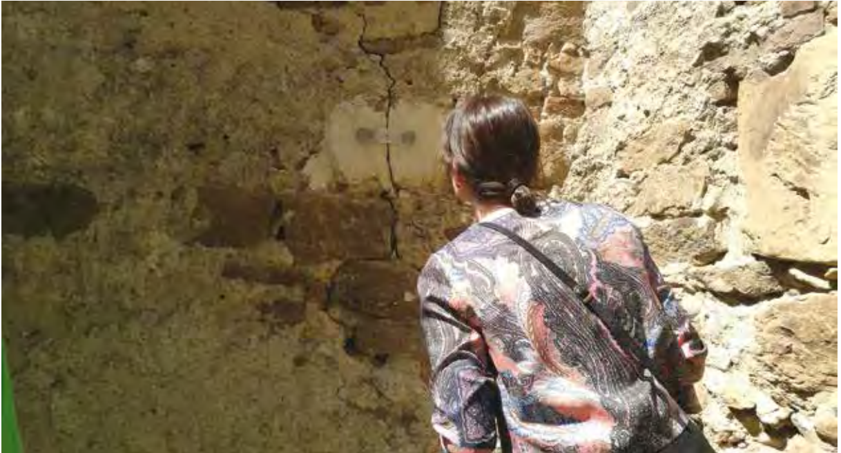
A marker for recording evolution of structural cracks on the walls of the fortified church of Alma Vii. While restoration works are, for now, exceeding the capacity of the community to undergo, the condition of the fortified church is strictly monitored and maintained.
