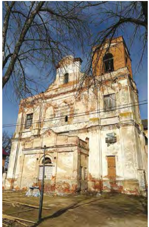
Architectural sketches and current condition of the Jesuit Church in Mstislavl, Belarus. The degree of degradation poses significant challenges to the local team in identifying the proper architectural and construction solutions for its renovation.
